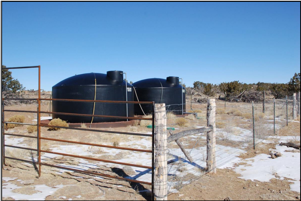
Storage tanks on the pipeline
