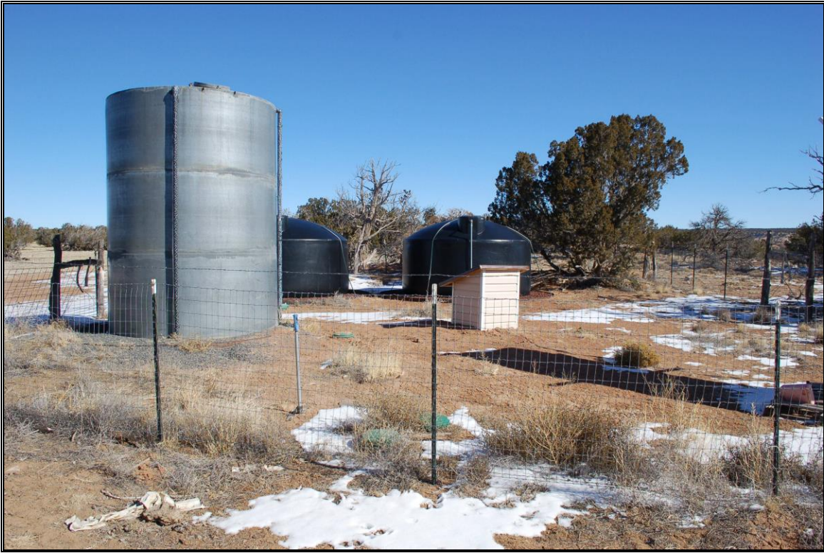
Livestock well with solar pump & storage tank
