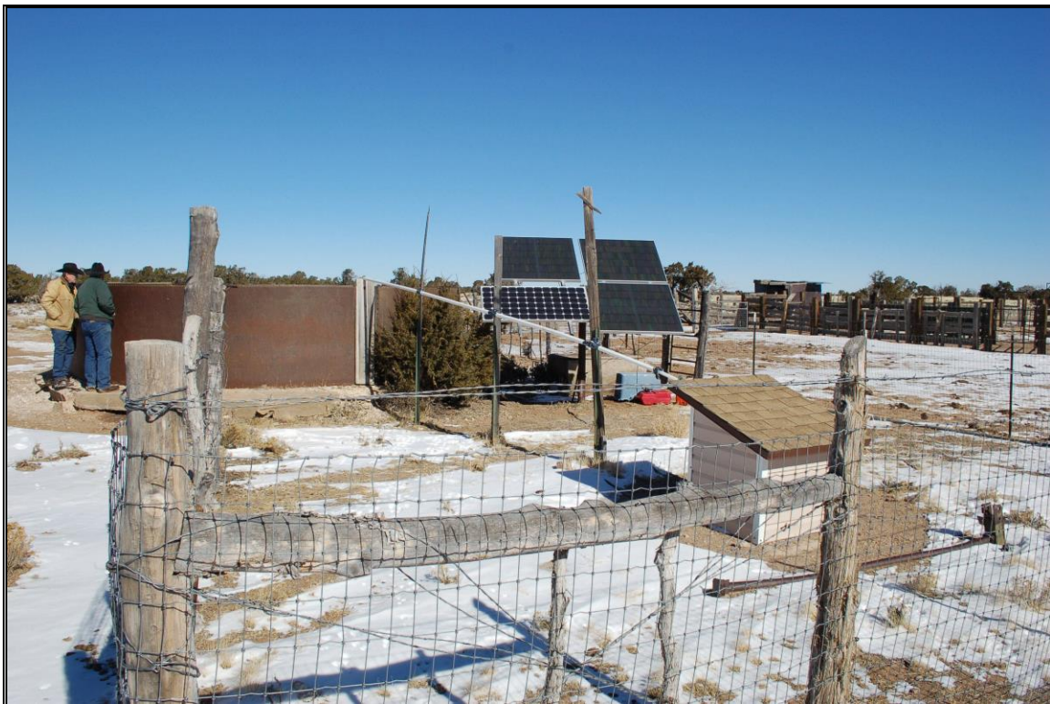
Livestock well with solar pump & storage tank
