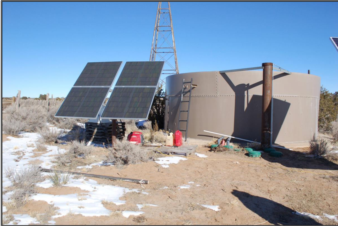
Livestock well with solar pump & storage tank
